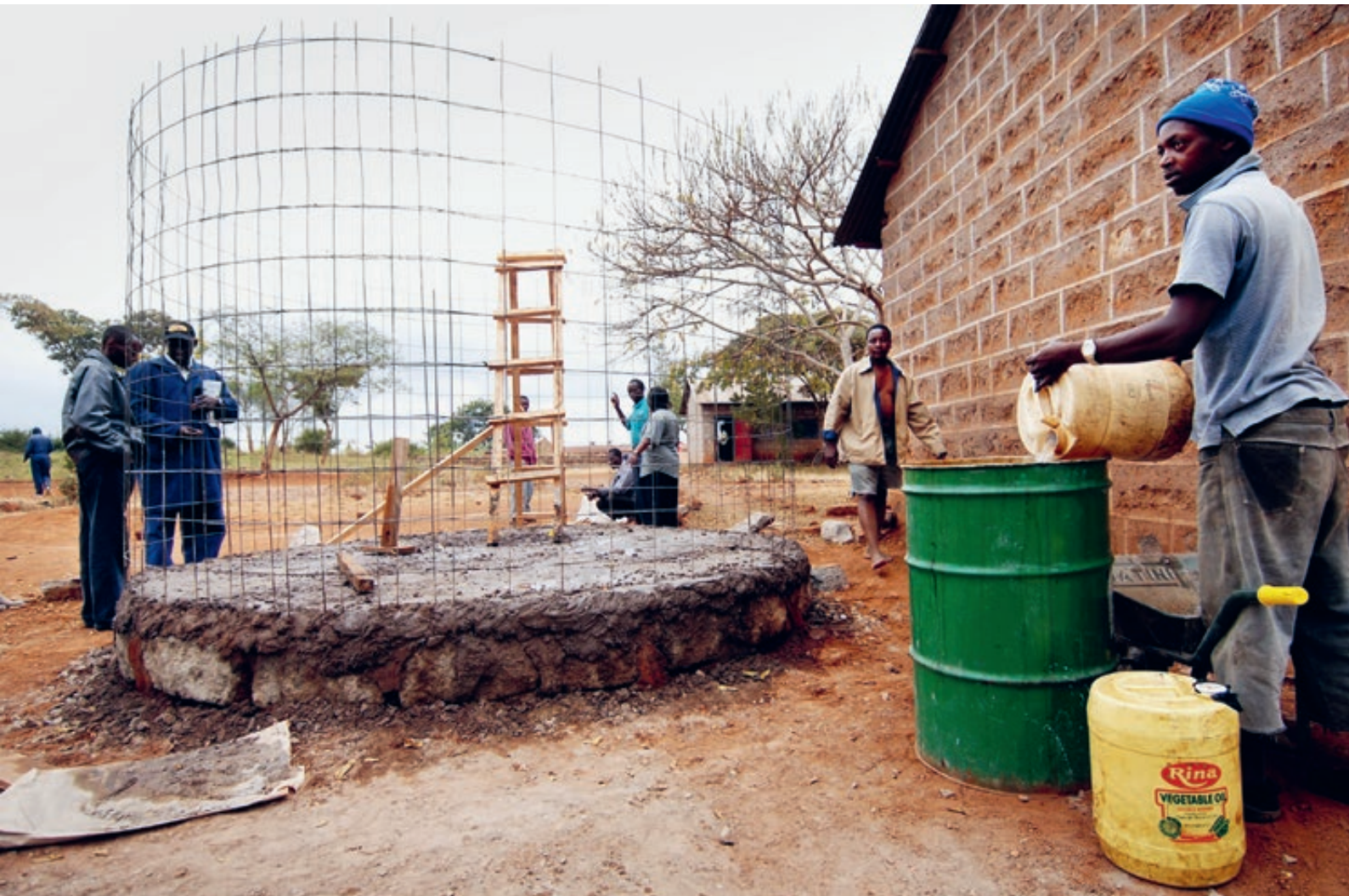
Students constructing a water tank in a rural village in Kenya contributing to improved water supply.
