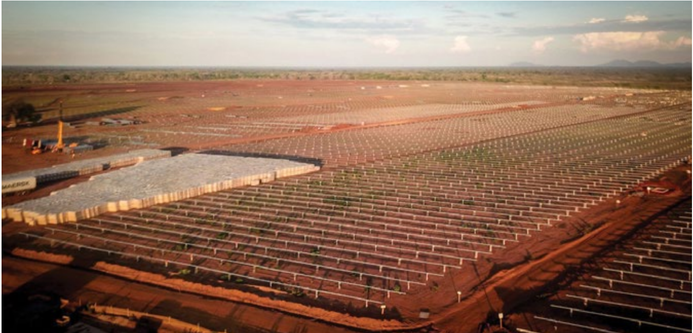
A 60 MW project being built in Malawi. The project creates 300 local jobs and is expected to contribute significantly with 20 percent of Malawi's current installed capacity.
